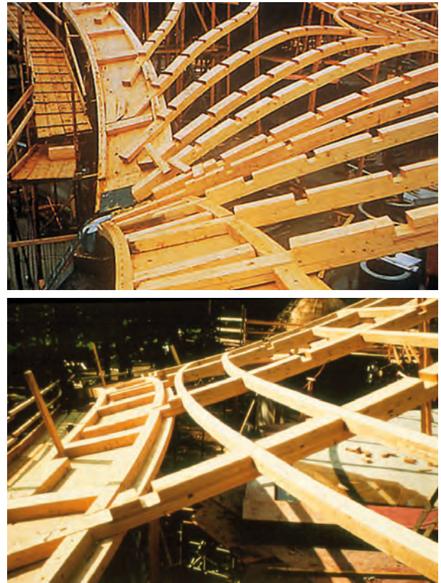
Figure 12.9 (top) Meridian ribs with cross lap joints, attached to the edge beam, and (bottom) overlaid with the annular ribs
