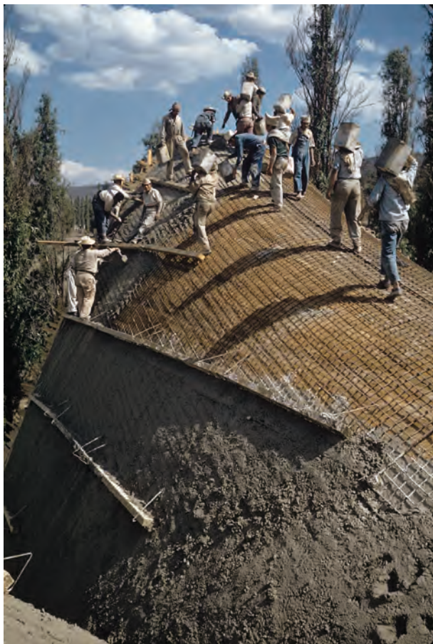
Figure 20.15 Laborers placing buckets of concrete on the shell for Los Manantiales Restaurant (see Fig. 20.10)
