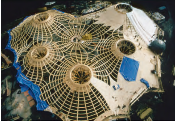
Figure 12.7 Construction site with all ribs assembled and placement of covering boards and sheeting
