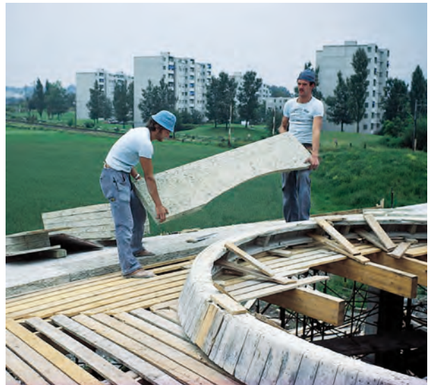
Figure 20.18 Leuzlinger Sons Building, 1979. Isler standing beside glued laminated timber arches, and formwork of fibreboard insulation placed on wooden boards
